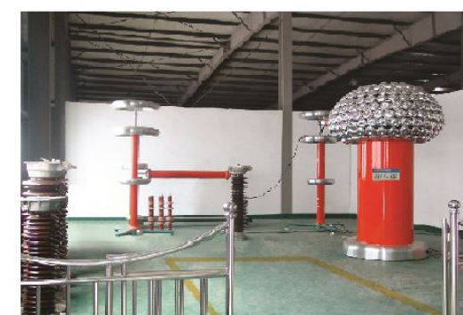
Power frequency withstand voltage inspection
